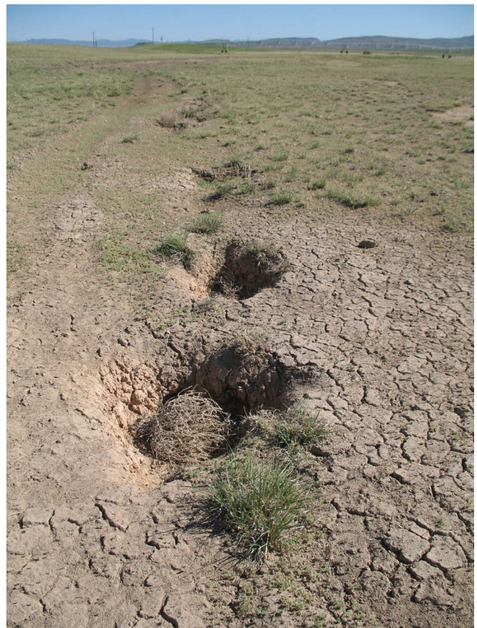
Figure 25. Sinkholes aligned along the EGWF1 fissure (view is to the northwest). Photo taken in May 2009.
